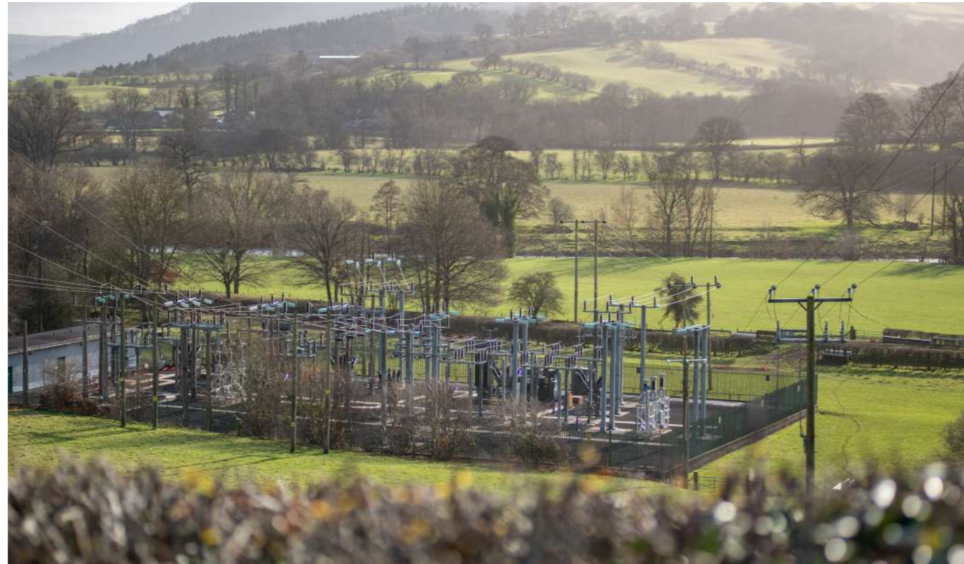
Existing Builth Wells substation which provides an indication of the type of development the switching station will be.
